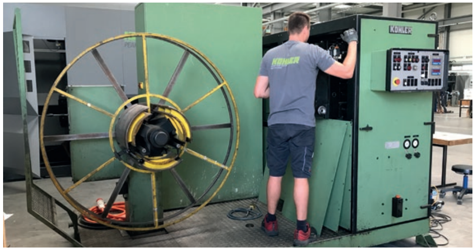
Retrofitting is often the right solution, as with this 30-year-old strip leveling line. To enable the customer to still keep using the proven and familiar technology economically over the long term, KOHLER modernized and overhauled the line in Lahr, bringing it up to the latest safety and control standards.
